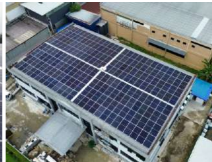
Project Name : Malaysia Tofu Factory BIPV Project Installed Capacity : 145KW
