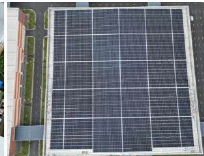
Project Name : Qianzhiya Sanitary Products Co., Ltd. (Hubei) Installed Capacity : 2.2MW
