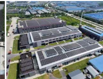
Project Name : Anhui Yunyan Food Technology Co., Ltd. (Ningguo, Xuancheng, Anhui) Installed Capacity : 1.7MW
