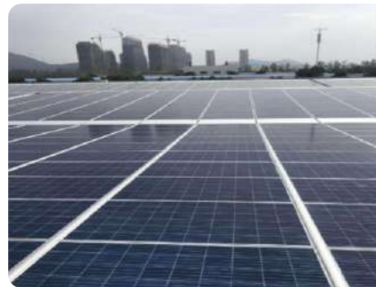
Project Name : Weiman Aluminum Technology Co., Ltd. (Chizhou, Anhui) Installed Capacity : 5.9MW
