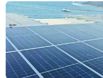
Project Name : Sanya, Hainan Coastal Rooftop Solar BIPV Project Installed Capacity : 200KW
