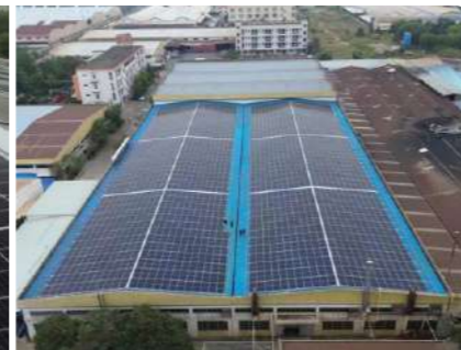
Project Name : Fuhua Industry Co., Ltd. (Pengjiang, Jiangmen, Guangdong) Installed Capacity : 1.0MW
