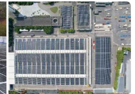
Project Name : GiantKONE Elevator Co., Ltd. (Huzhou, Zhejiang) Installed Capacity : 3.7MW
