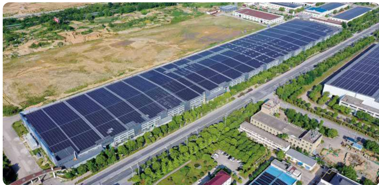
Project Name : Luffy Magnesium Technology Co., Ltd , (Anhui) Chizhou, Anhui Installed Capacity : 8.7MW
