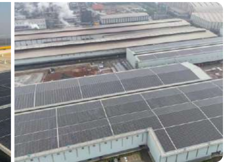
Project Name : Anhui Guihang Special Steel Co., Ltd. (Guichi, Chizhou, Anhui) Installed Capacity : 20MW
