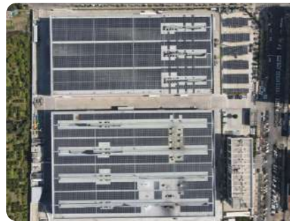
Project Name : WMF Household Products Co., Ltd., (Zhejiang) Yuhuan, Zhejiang Installed Capacity : 5.0MW
