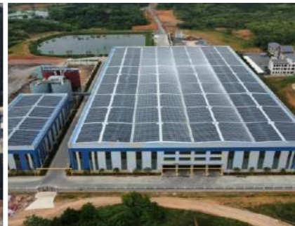
Project Name : Huicheng Co., Ltd. (Chizhou, Anhui) Installed Capacity : 5.9MW
